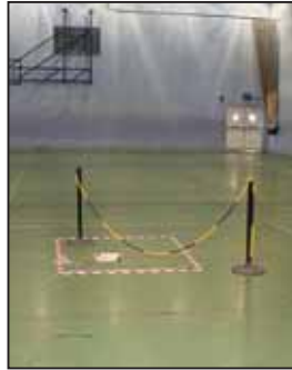
The sports hall at de Stafford showing the unsafe area of the floor.
