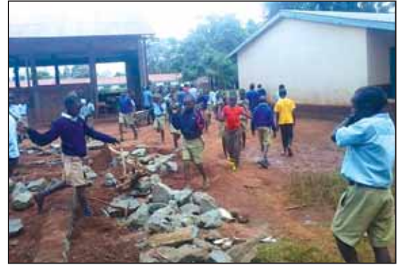
St. Joseph's pupils start work on building the library's foundations in Kimilili.
