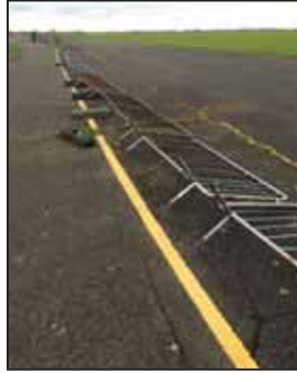
The existing unsightly crowd barriers that present a risk to safety when fallen down.
